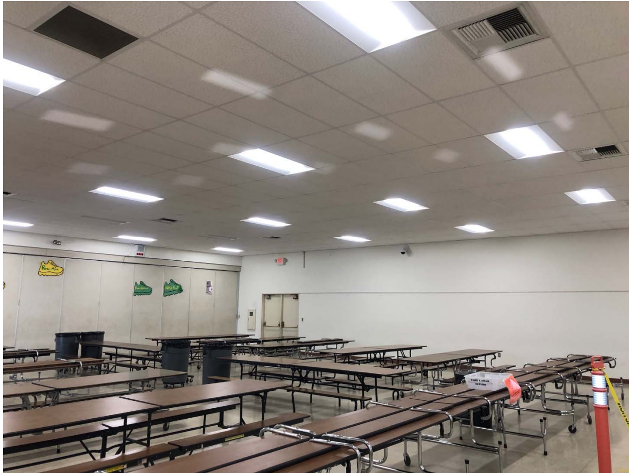
T-Bar and LED Lighting – James Monroe Multi-Purpose Room
